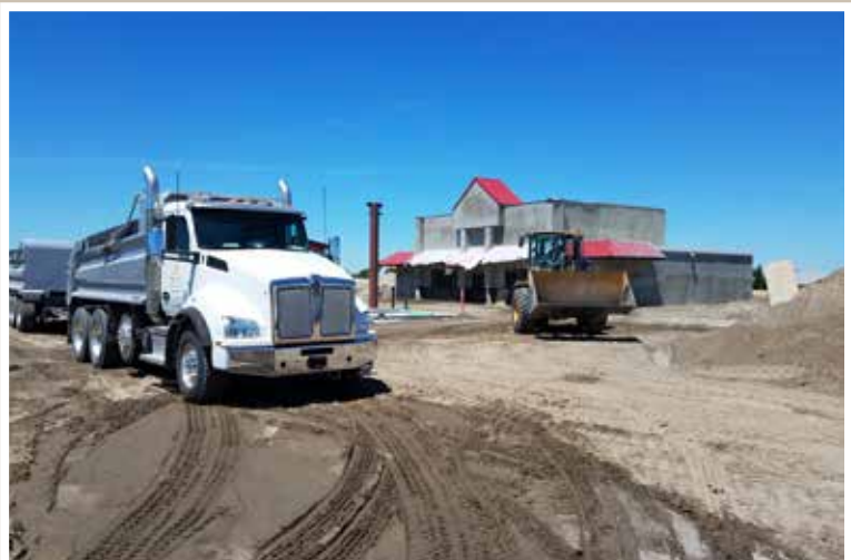
Elvin with Anchor Hauling was giving the C&E crew a hand on the site work for a new Pasco gas station going in.
