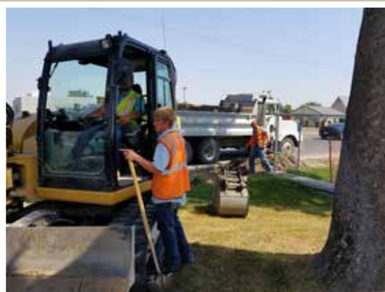
Next time you are driving by Pasco High on Court Street, check out their new sidewalks! Our thanks to the crew in this photo for making it happen.
