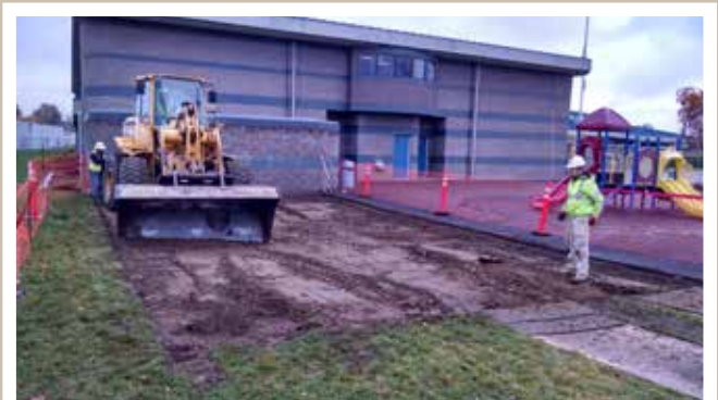
Travis is keeping a close watch so we don't over cut the sub grade on a small project for the Pasco School District. They are adding some paved playground space.
