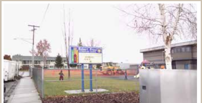
Lucky kids! Who needs a playground when you can watch construction equipment at work?
