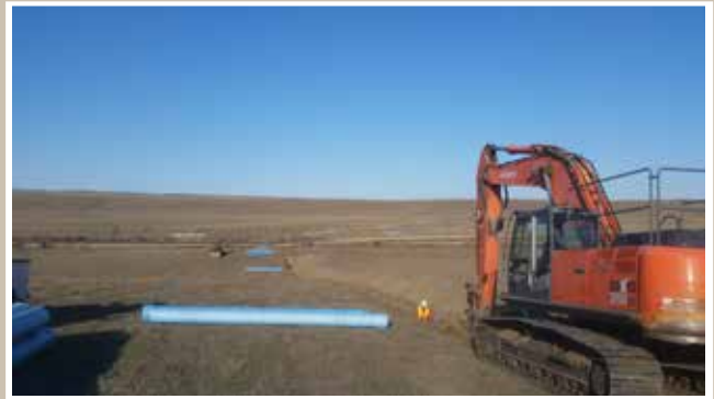
Cwentin and crew hard at work laying new irrigation main near Plymouth, WA on one of the rare, but much appreciated, sunny days this time of year.
