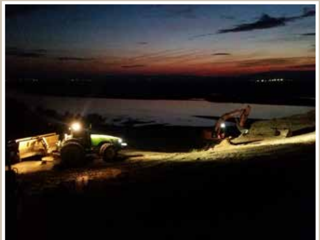
Moving dirt and cutting out a substantial pad for a new house overlooking the Columbia. We are thankful for lights on these early evenings!
