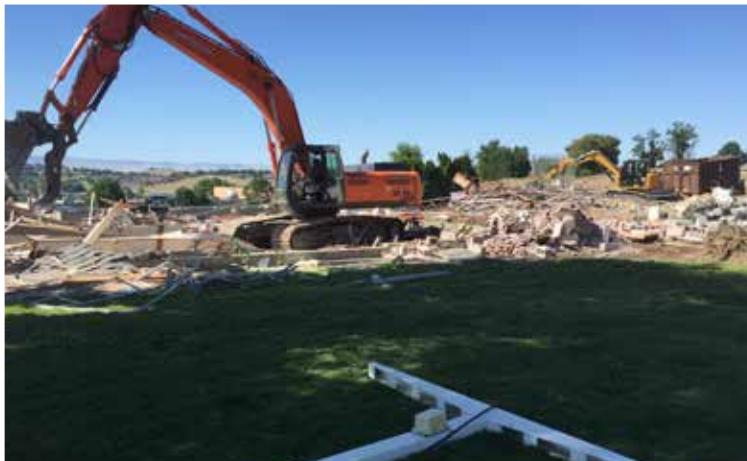
Another part of the PSD (Pendleton School District) project required we demolish the old gym.
