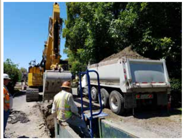
Nate takes a break from the bottom of a deep hole while waiting for the next sewer pipe to be set. Our project was extending a sewer main in Kennewick.
