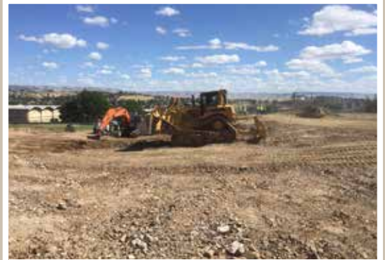
We have lots of pictures of the PSD project this month. Here the D8 is ripping rock on a beautiful day in Eastern Oregon.
