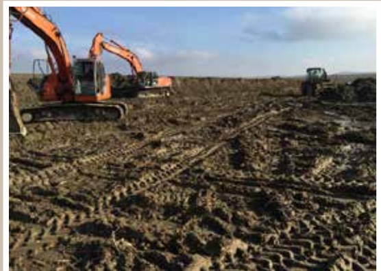
Mud, excavators and pipe to lay! Who says you can't live the dream?
