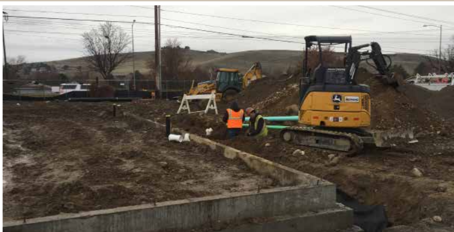
Nate and Lonnie tie in sewer to the new Fire Station in Kennewick, with the aid of Petunia. Petunia is the small excavator in the foreground which, according to Robert, is only good for picking petunias. (Hence the nickname.)
