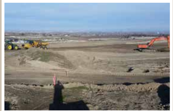
The start of a large pond with well over 20,000 yards moved to start. The view is overlooking Kennewick.
