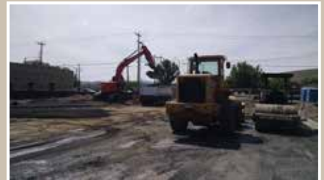
Elvin paused while being loaded to snap this photo of the progress at Kennewick's newest fire station. Their parking lot will be done soon!
