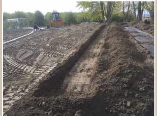
Here is a drain field going in for a septic on a new house. Our thanks to the Cutler family for inviting us to be a small part of their project.
