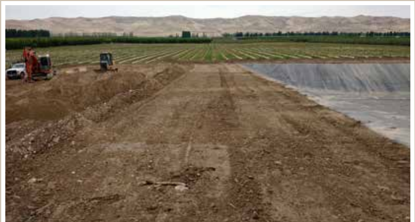
Here is the Mattawa frost control pond lined, graded and almost done! Also a cool view of Eastern WA orchard and hills!
