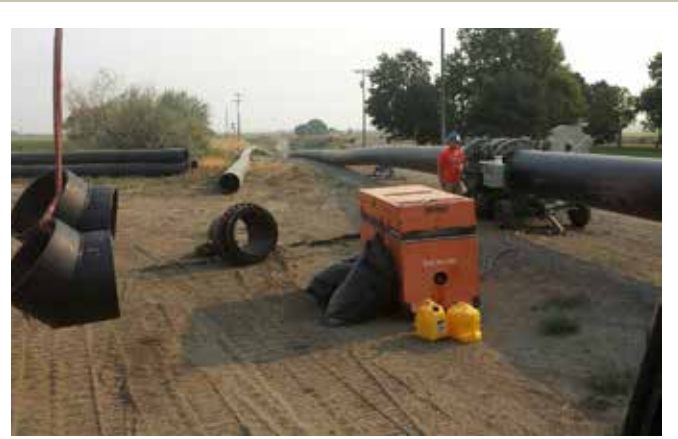
Here we are fusing 32" HDPE pipe for the South Columbia Irrigation District. Our thanks to Devin from HD Fowler who was great to work with on this project.
