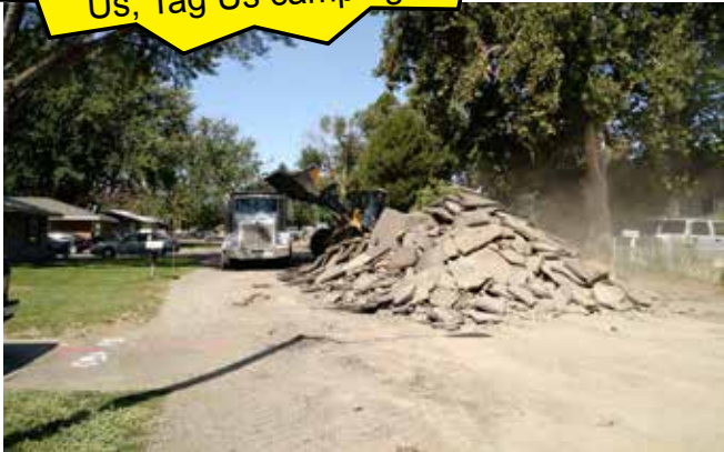
Out with the old, in with the new. Fifth Avenue in Kennewick is getting an upgrade. Phase 1 - Demo.
