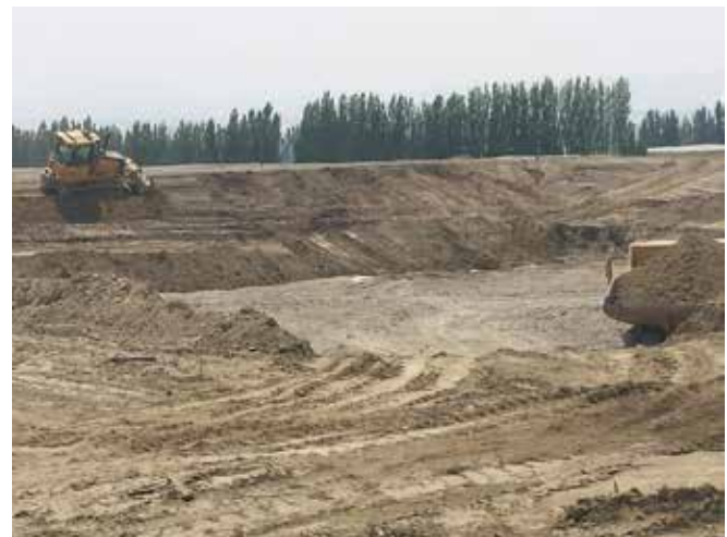
Sal, one of our skilled dozer operators, cuts the side slope with precision.
