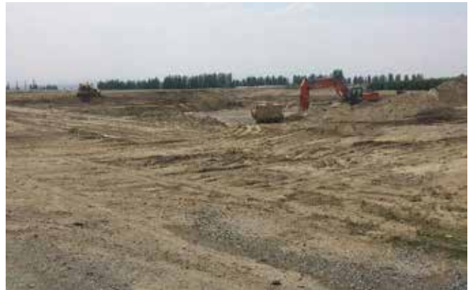
These three pictures are of a frost control pond we recently finished near Mattawa.
