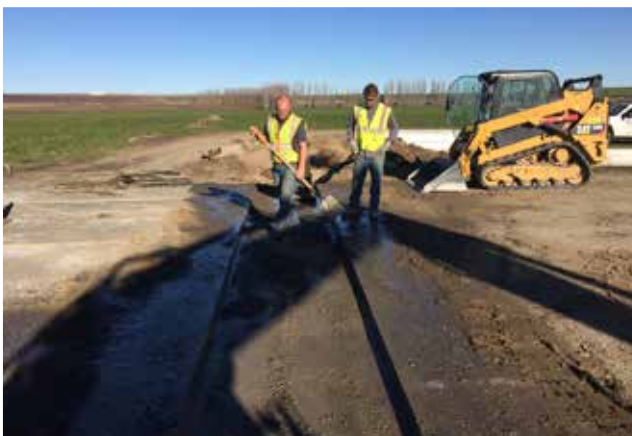
Cwentin and Matt put the final touches on the gravel before paving back a road crossing in North Franklin County.
