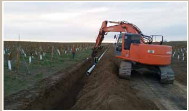
Sal, Edgar and Nate laying 12" mainline way out in Washington wine country. This main will provide irrigation water to another large block of grapes.
