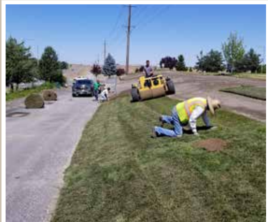
Putting the final touches on a new asphalt bike/walking path in Richland. Our thanks to the City of Richland for letting us partner with them on this project.
