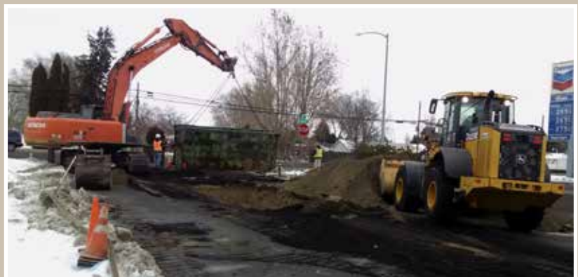
If you drive on Road 38 in Pasco, you may notice less puddles! Our crew is installing a new storm system for the City of Pasco.
