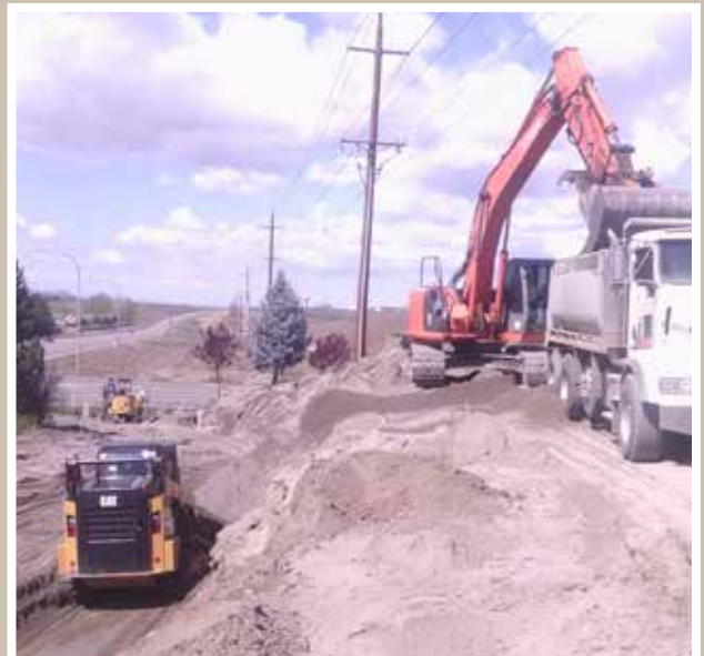
C&E crew prepping for a retaining wall to hold this bank back along Highway 240 where we are building a new bike path.
