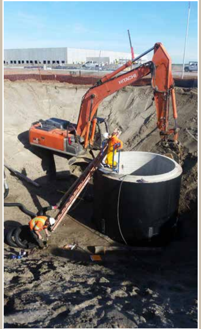
Jack & Nick working on installing a 12' wide by 30' deep concrete wet well for a sewer lift station in the King City area.
