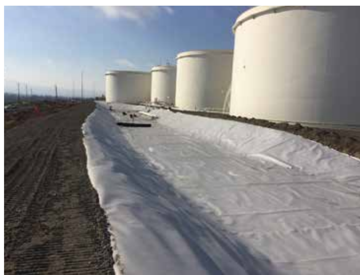
Here the C&E team is helping Tesoro improve their existing containment. The existing was earthen with a clay core, while the new is HDPE. While this picture isn't super exciting, we enjoy helping make infrastructure safer!
