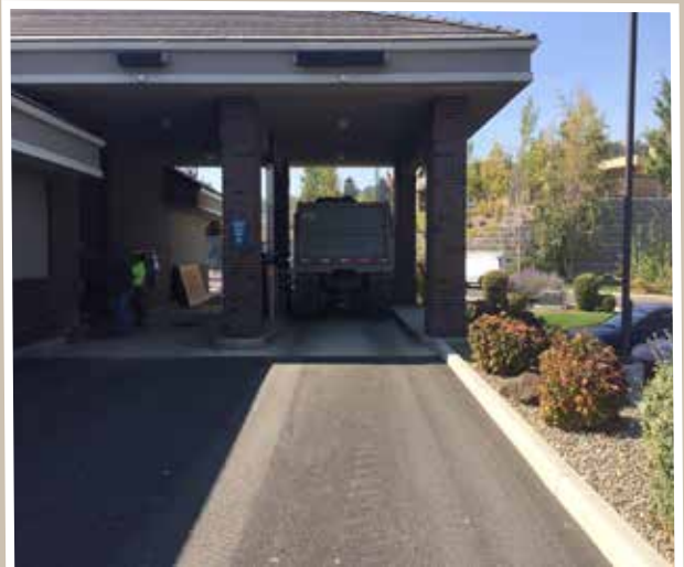
I would like to make a deposit...yes, about 12 yards of dirt. Improving drainage around a Gesa Bank in Sunnyside was the task. The photos are just a side benefit.
