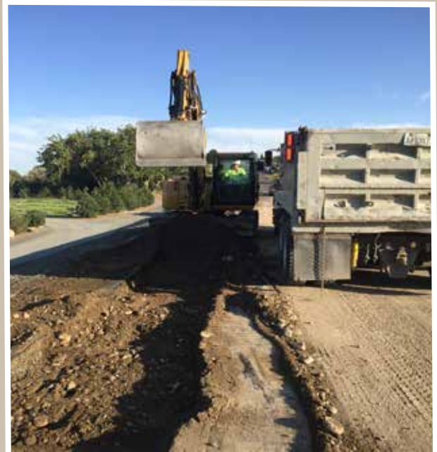
Eric operates our 308 Cat excavator, sub-grading the trench and getting it ready to place gravel.
