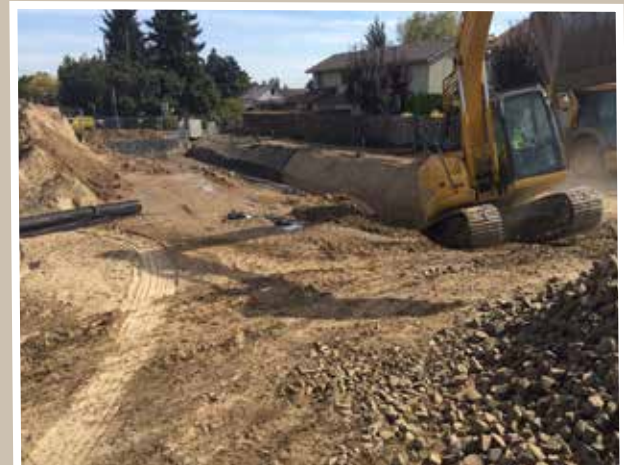
Rudy climbs our 140 excavator out of the hold while digging a huge infiltration trench for storm drainage at a soon to be brand new Gesa branch in Yakima.
