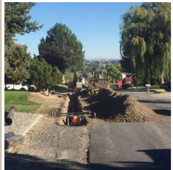
High on the south hills of Kennewick, the C&E team is installing a new water main and services for the local residents of the neighborhood.
