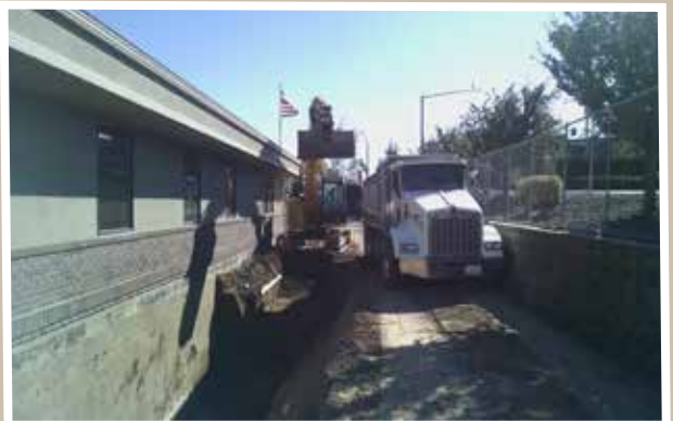
Same site as above in very tight working conditions. But Robert and team were up to the task and the building is still standing so we are calling it a win.
