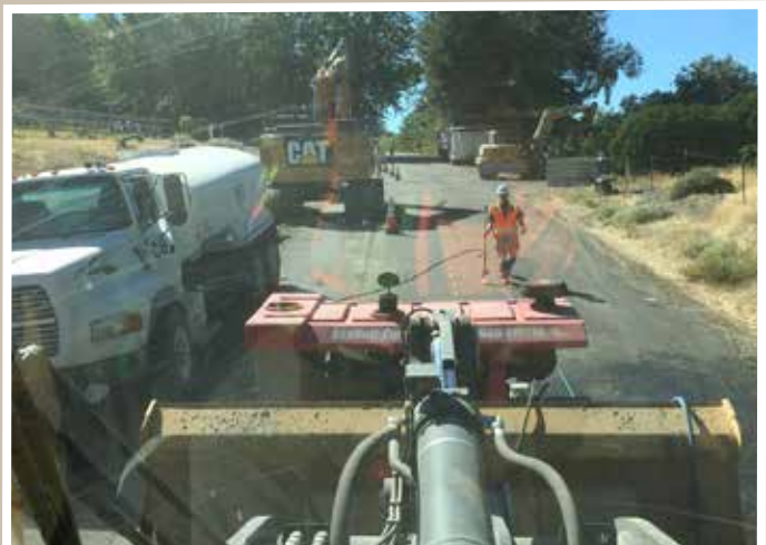
A look from the operator's seat of a loader with an asphalt zipper mounted to the bucket. The zipper grinds a 4' wide path through the asphalt, preparing the way for the trench to follow.
