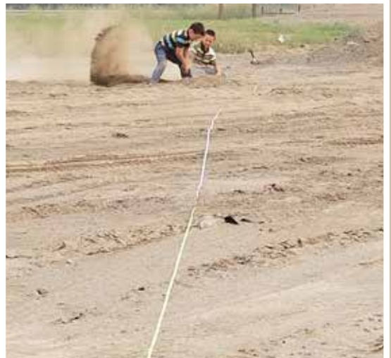
A couple of young and talented diggers from Aquatech were helping Jake layout the foundation on C&E's new office. A small pile of dirt was in the way but they had a solution!
