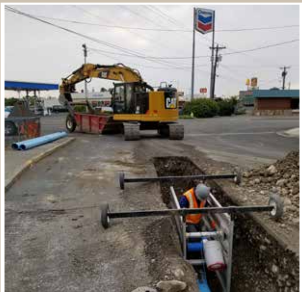
Edgar and crew work on installing a new water main in Kennewick.
